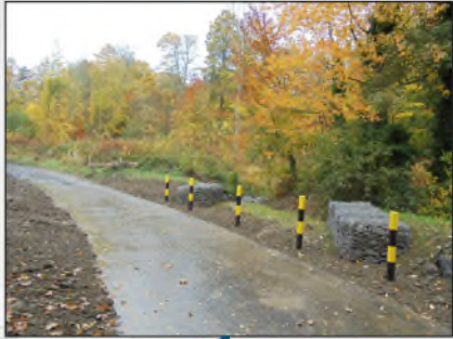
New overflow spillway which during very high flow events will divert excess flow onto Corby Linn Road, protecting Ravensheugh House from flooding
