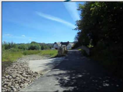
New ramp and channel to redirect excess flow back into the burn
