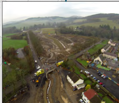
Angles Field flood embankments, re-meandered burn and new A707/A708 junction during construction
