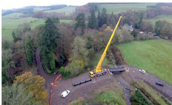
Above: Temporary Bridge being constructed at Corby Linn, November 2014. Courtesy of G. A. Talbot
