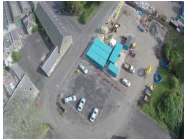
Above: Advance Works Site Compound on South Bridge Street.. Taken in summer 2014. Courtesy of G.A. Talbot.
