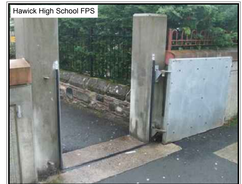
Aluminium flood gate
